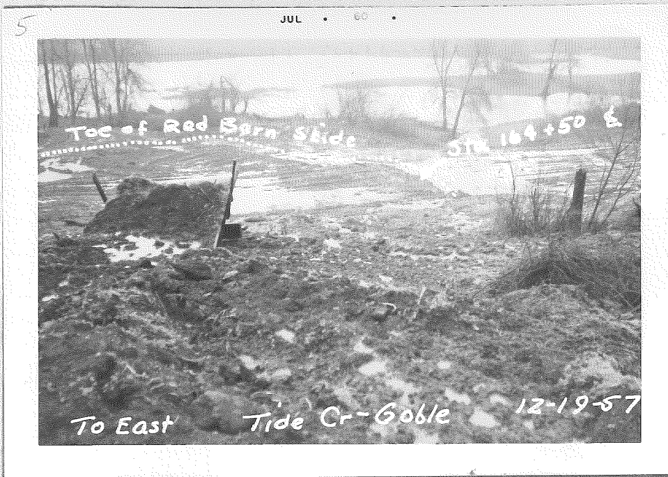
Photographs 6 to 10 show the surface cracks and settlement in the vicinity of the Red Barn.
